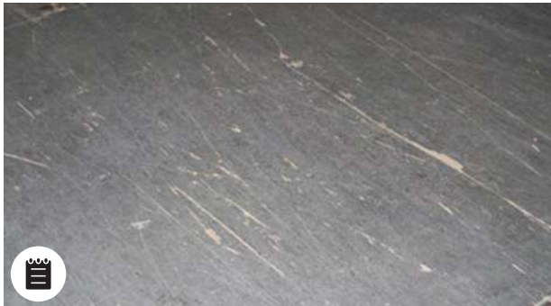
Flooring: Slight deformation, superficial wear
