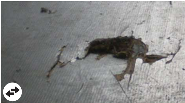
Flooring: Deformations or perforations within economic repair
