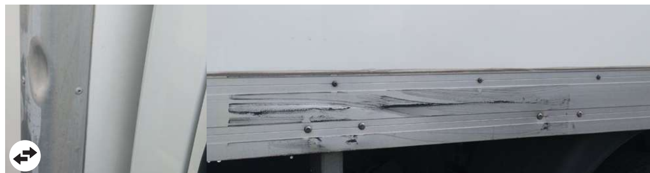
Underbody side profiles: Deformations within economic repair
